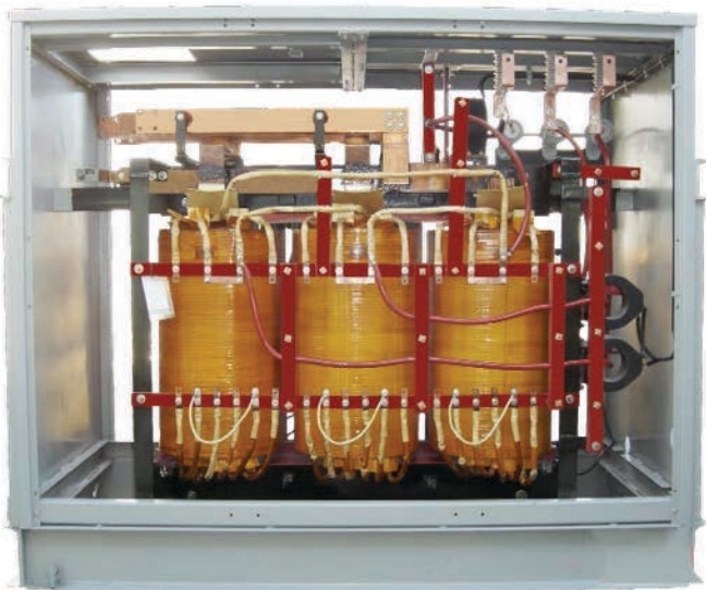
504087 H&H Trans., 2000 KVA, 550/7200-600Y//600Y
