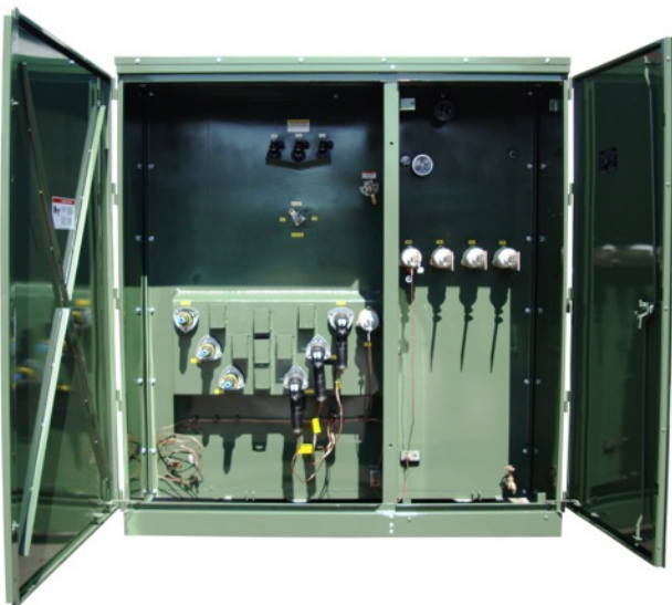
709190-1 H&H Trans., 2500 KVA, 24940GRDY/14400-4160Y/2400
