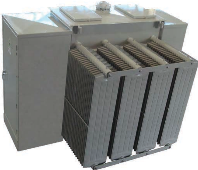
1108112 Arizona Electric, 3000 KVA, 4160-480Y/277
